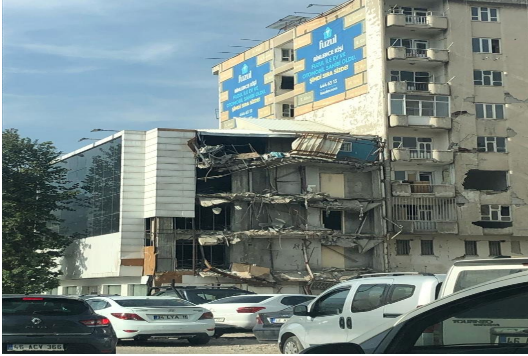
Figure 2: A Commercial Property and Residential Building Severely Damaged by the Earthquake in Kahramanmaraş
